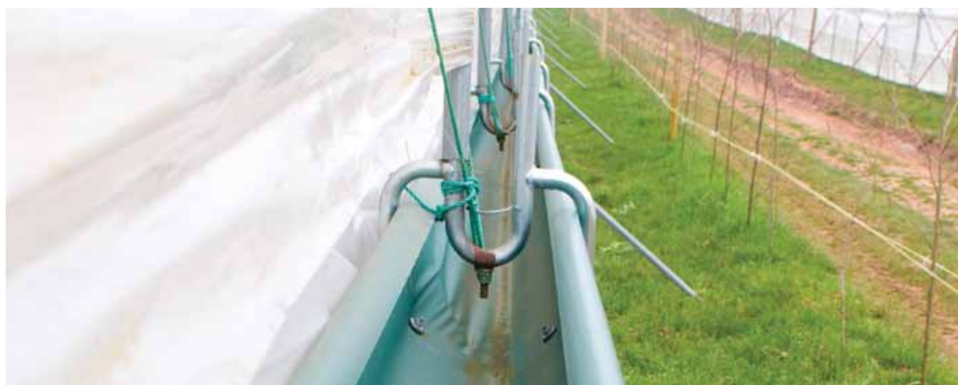
Good guttering is vital to capture rainwater
